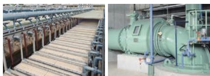
● Water treatment plants ● Pumps
