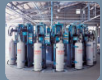
LPG FILLING SYSTEM
