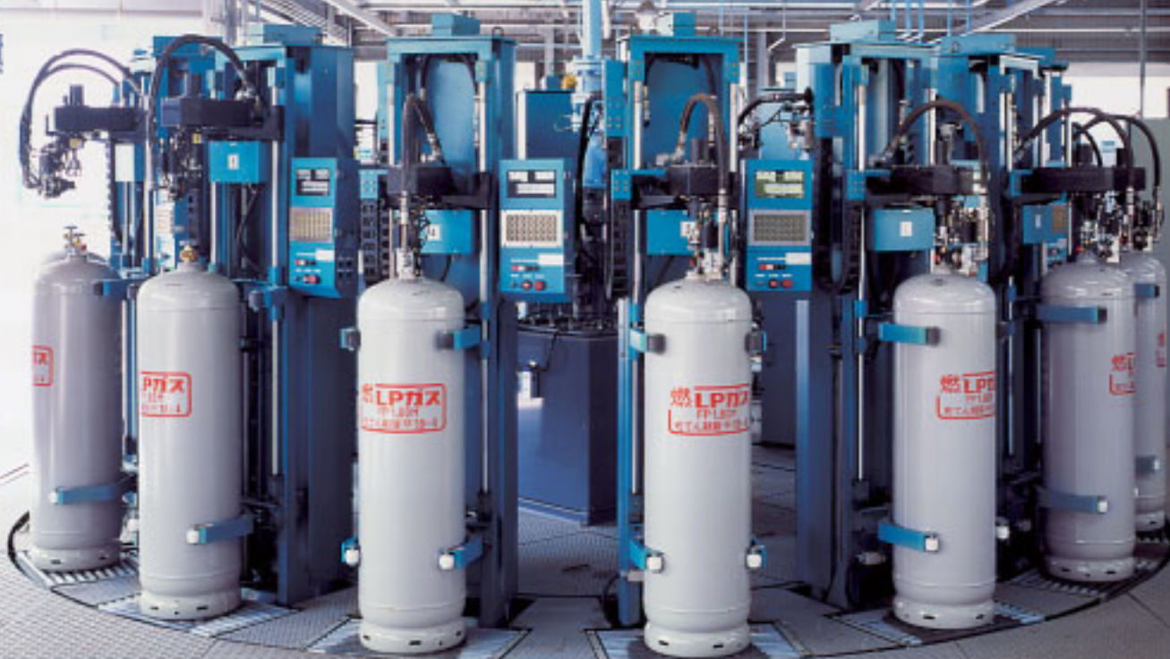
LPG FILLING SYSTEM
