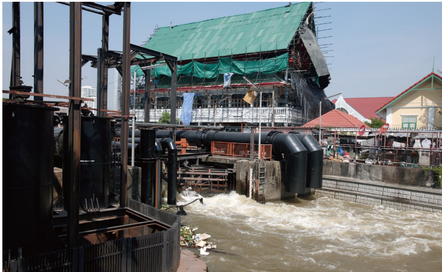
Large quantities of water pour in from the Chao Phraya River through flood gates. Several waterways spread across the entire city of Bangkok.
