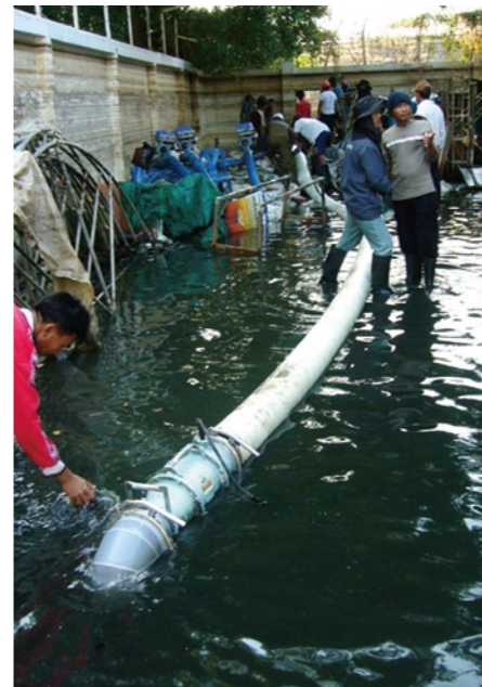
Draining water at the Nava Nakorn Plant
