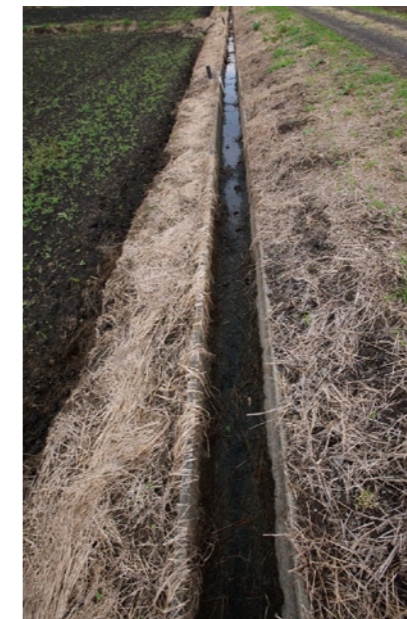
Demonstrations of desalination using rainwater without the need for irrigation channels were suggested by Kubota. (photo taken on October 17, 2011)
