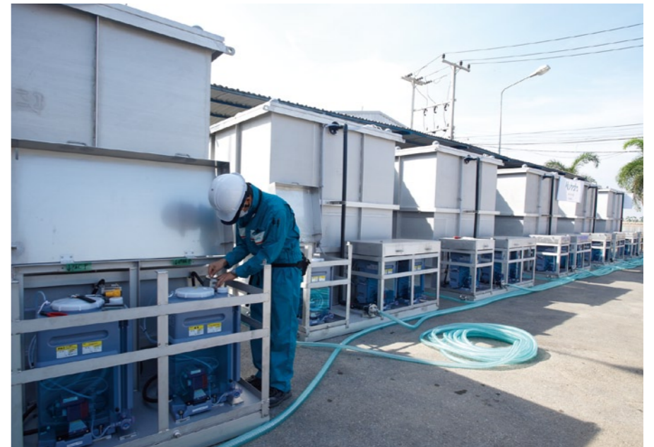
Water purification unit with power generator (FILCERA)
