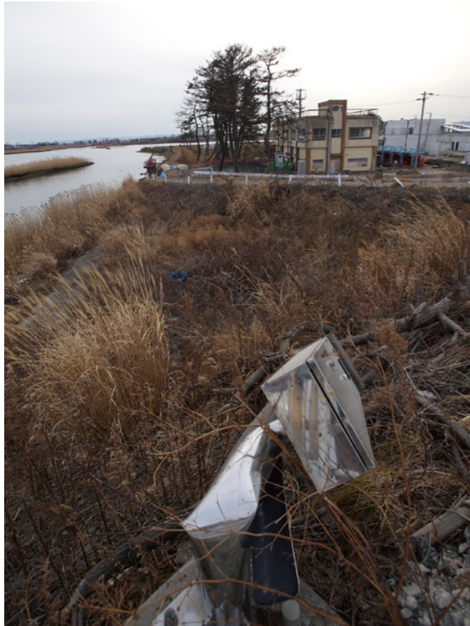
Tsunami-hit drainage pump station in Natori City, Miyagi Prefecture. It has since been repaired and is now in operation.
