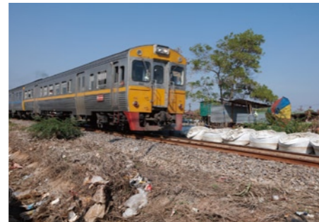
“Big bags” protect railway tracks from the floodwaters. (north of Don Muang Airport)
