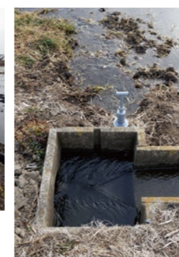
With the drainage pump station restored, an abundant supply of water poured into the field via the irrigation channel. (photo taken on February 17, 2012)
